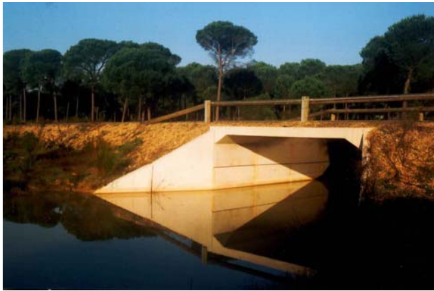
Figure 8: underpass on Villarmanrique – El Rocio road constructed for lynx passage, flooded (February 2004)
